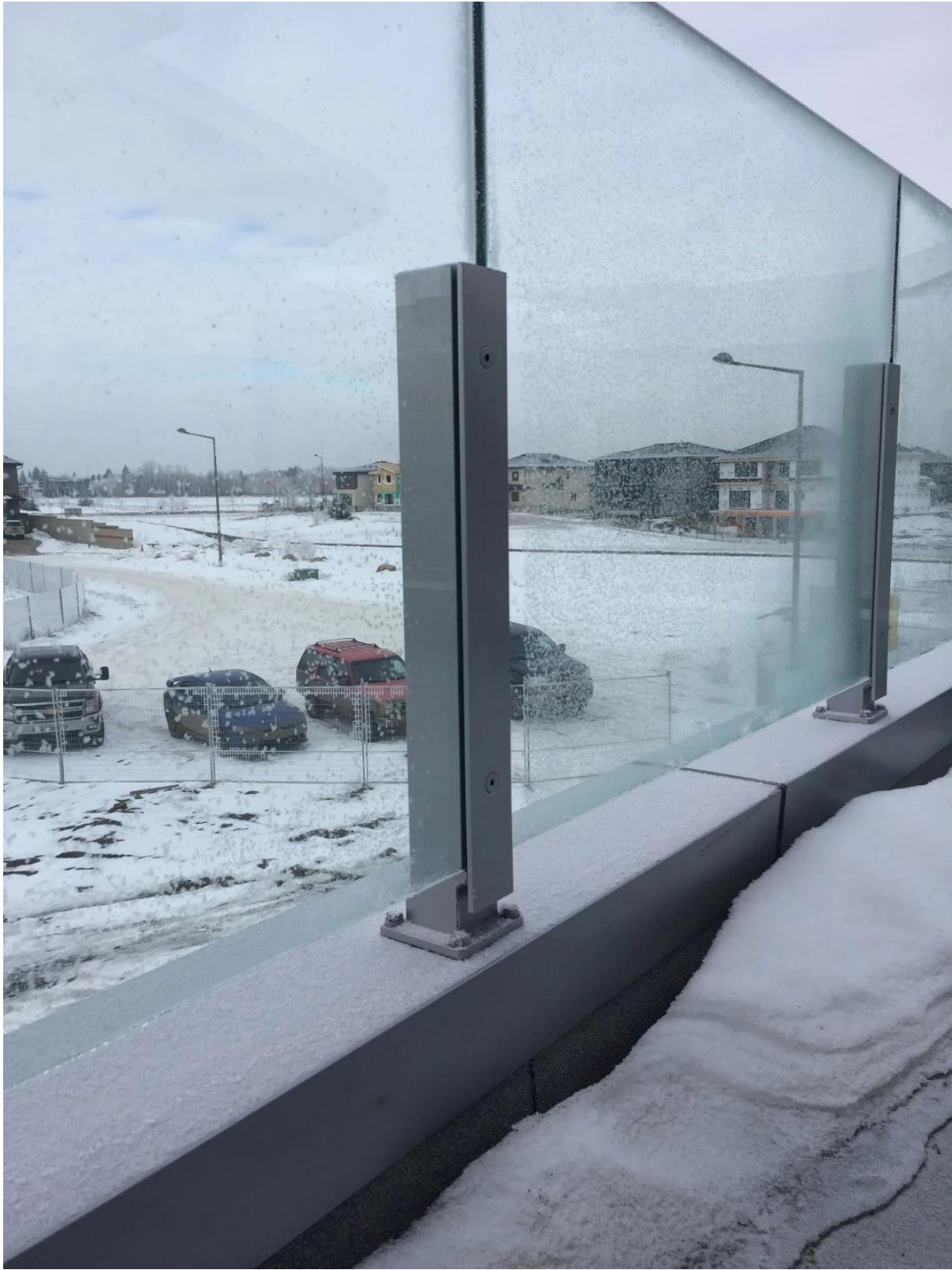
(4) Aluminum glass railing handrail post
