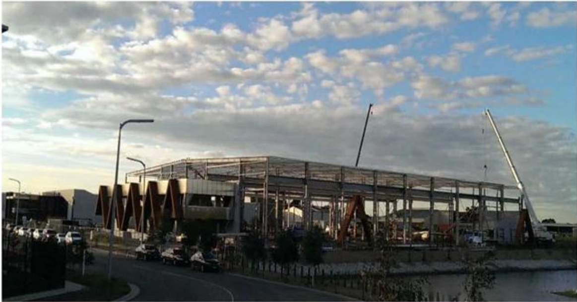
SS Front panel project for building in Australia
