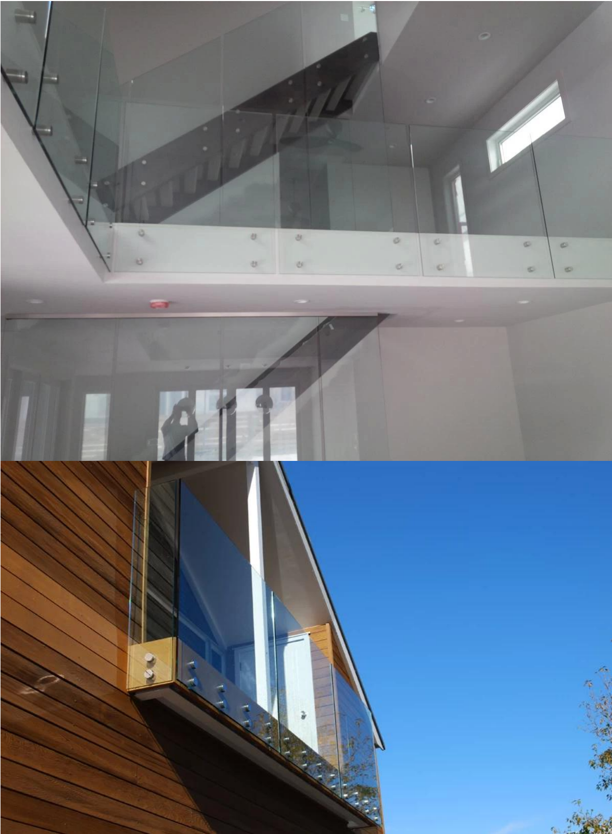
standoff + top handrail
