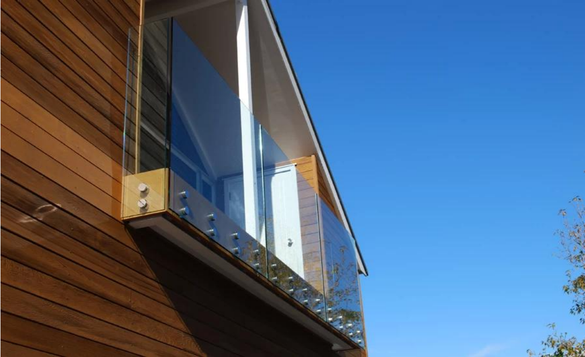
standoff + top handrail
