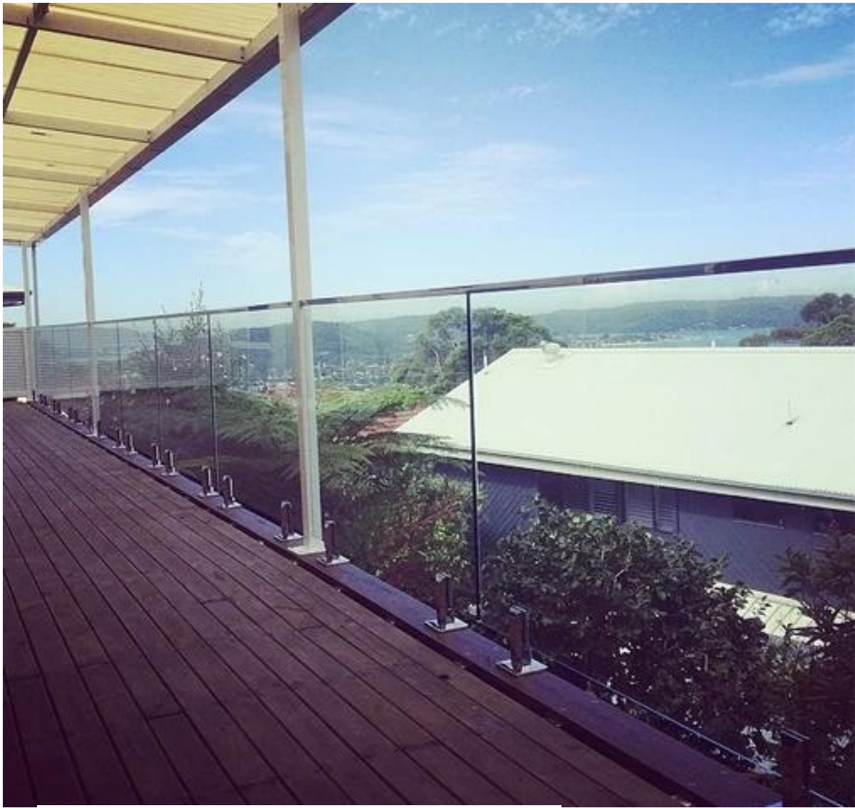
2). stainless steel top rails outdoor deck glass railings:
